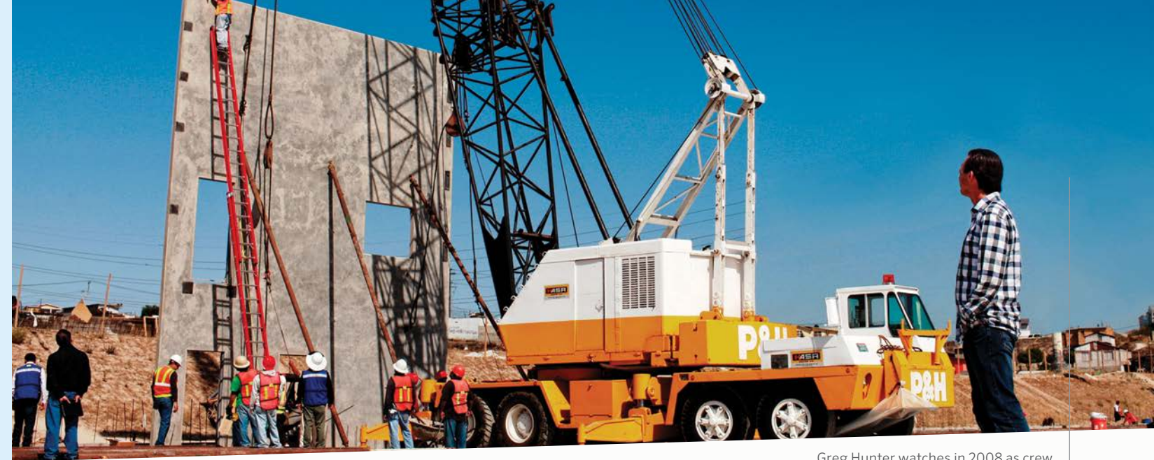
Greg Hunter watches in 2008 as crew members break ground on the new Hunter Industries distribution center, located at 1840 La Costa Meadows Drive in San Marcos, California.
